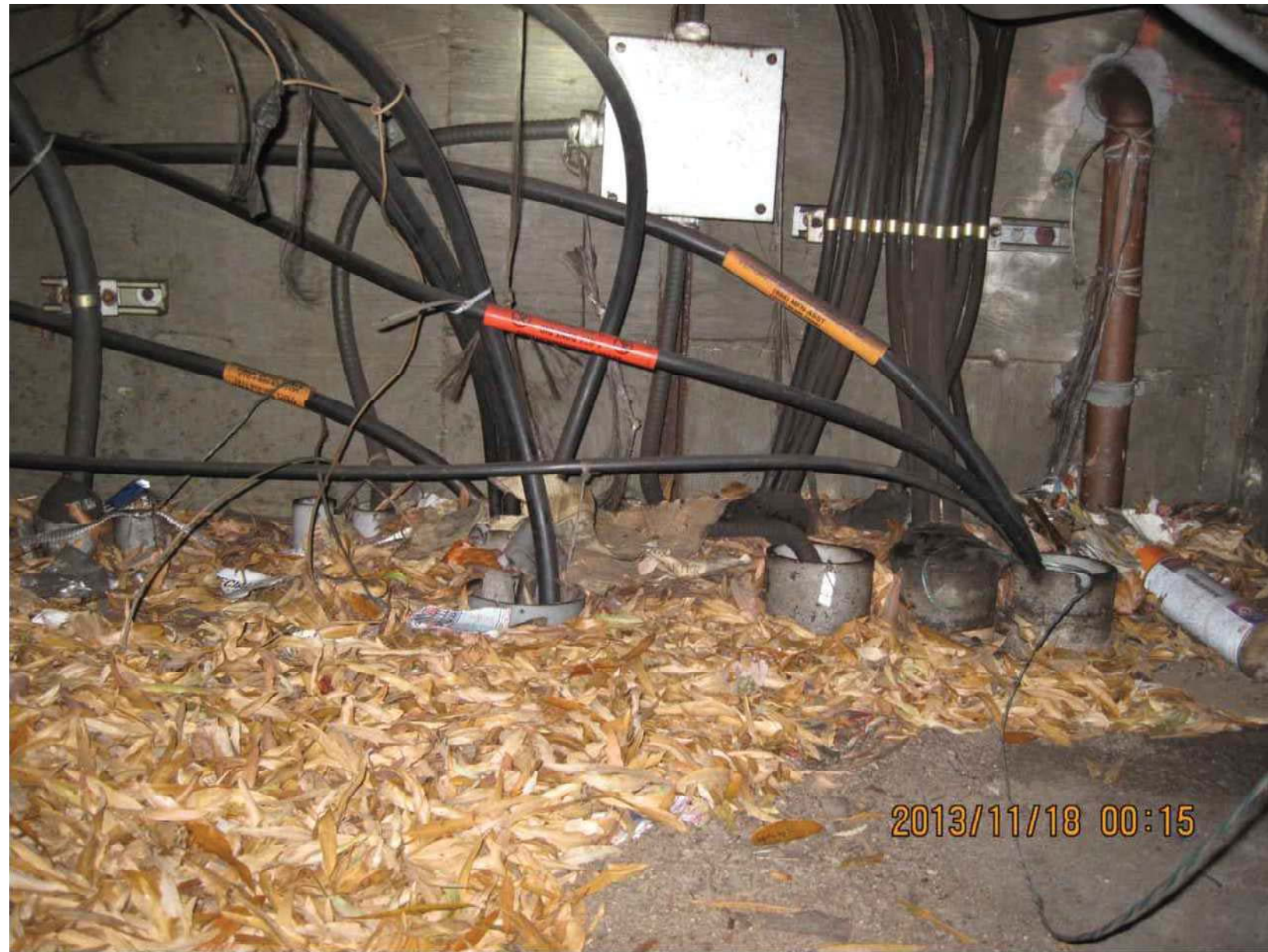
CONDUIT STUB UPS AND CABLE ROUTING AT END OF PLATFORM
