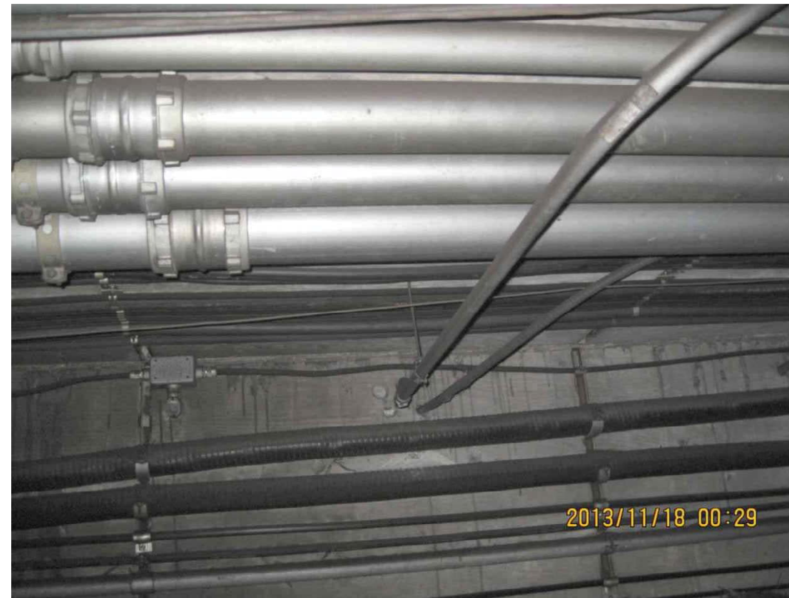
CONDUITS/CABLES UNDER PLATFORM OVERHANG AND OFF CONCRETE WALL
