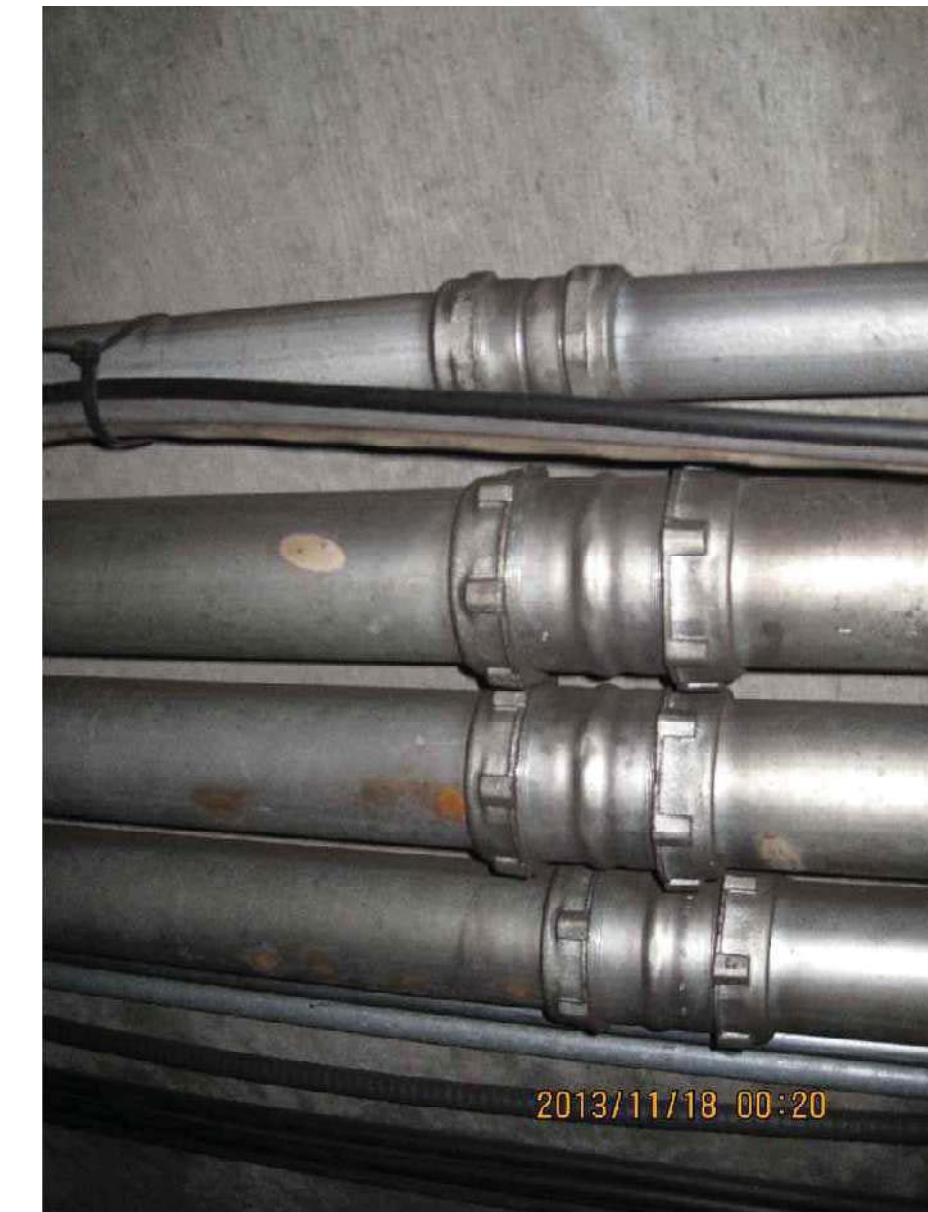
CONDUITS/CABLES UNDER PLATFORM OVERHANG
