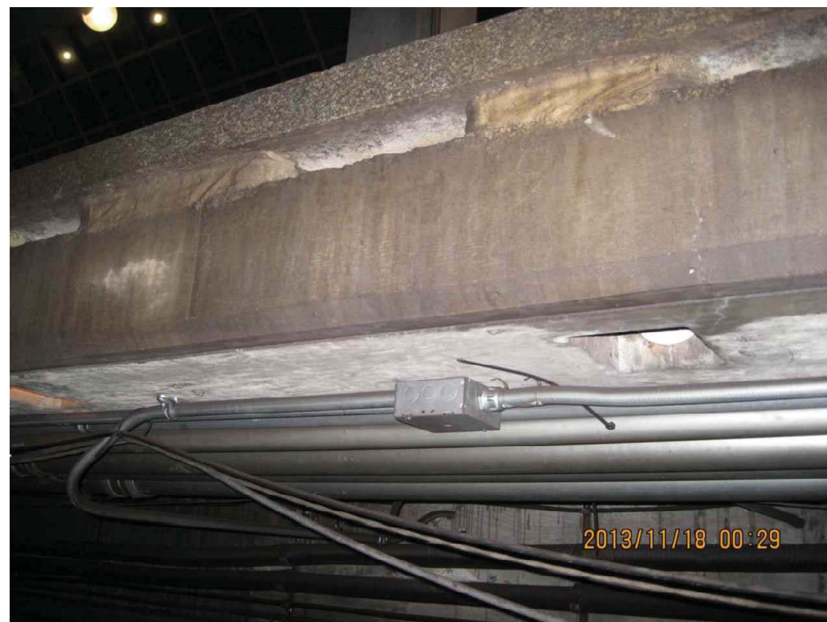
CONDUITS/CABLES UNDER PLATFORM OVERHANG
